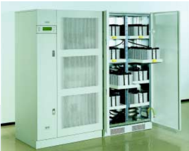
UPS with battery cabinet
