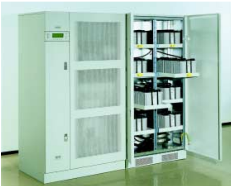
UPS with battery cabinet
