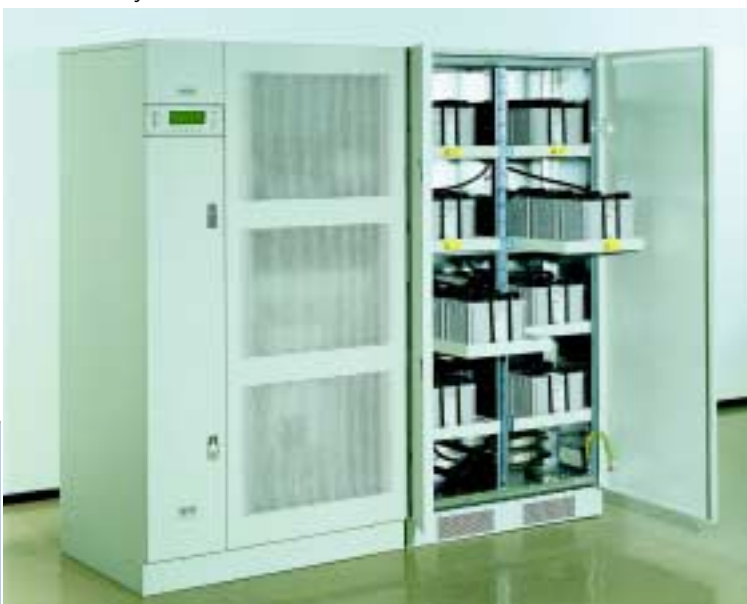
UPS with battery cabinet
